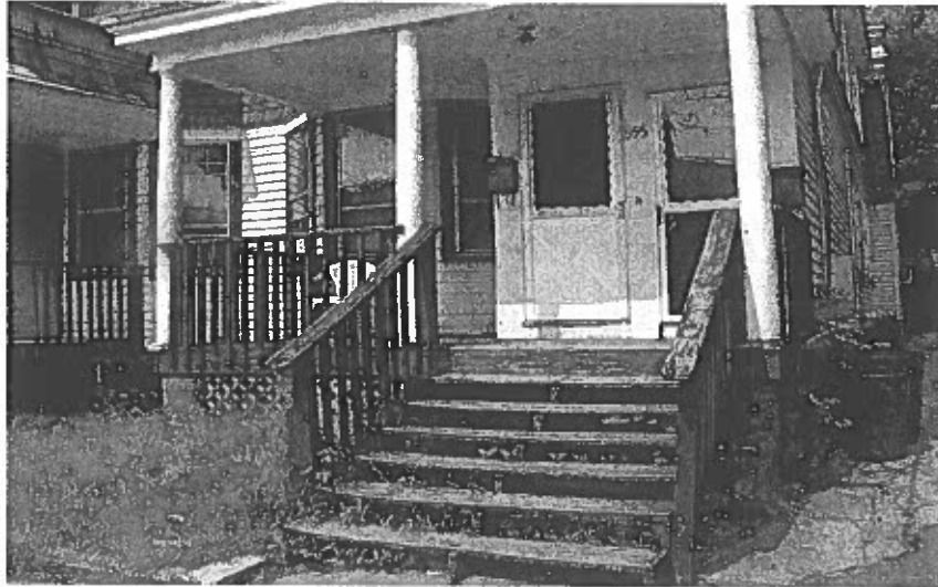
Building in Disrepair - 555-557 Whalley Avenue
